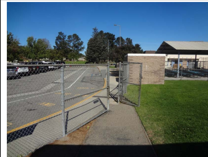
Photo -7 Kindergarten Entry The kindergarten entry to campus may have accessibility issues related to hardware and wheelchair clearances.
