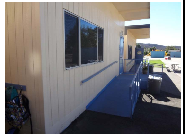
Photo -4 Numerous Portables There are numerous portable buildings, several of which are not DSA certified.
