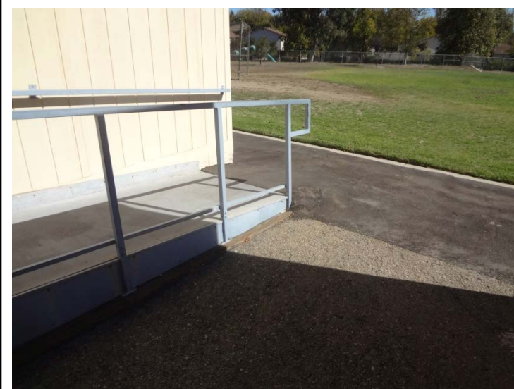
Photo -3 Accessibility Issues Campus wide accessibility upgrades may be needed to bring the campus in full compliance with accessibility standards.
