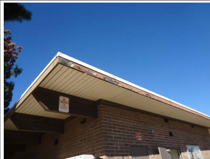
Photo -6 Maintenance and Repair Throughout the site there are areas that may require maintenance upgrades
