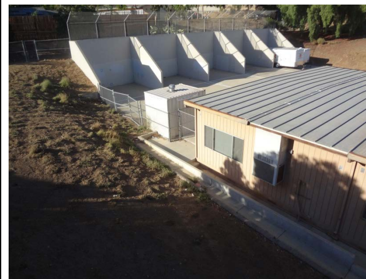
Photo -11 Safe Dispersal Path There is currently no paved pathway for emergency egress to the eastern portion of the field.
