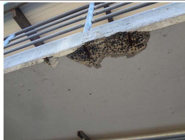
Photo -7 Elevated Classroom Walkway Spalling Concrete spalling occurs throughout the perimeter of balconies.
