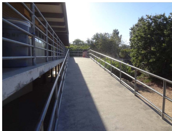
Photo -10 Elevated Classroom Ramp The ramp of the elevated classroom building is not compliant for wheelchair access. It is also a part of the egress path.
