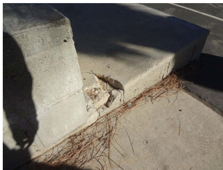
Photo -14 Concrete Deterioration There is concrete work that is needed throughout campus.
