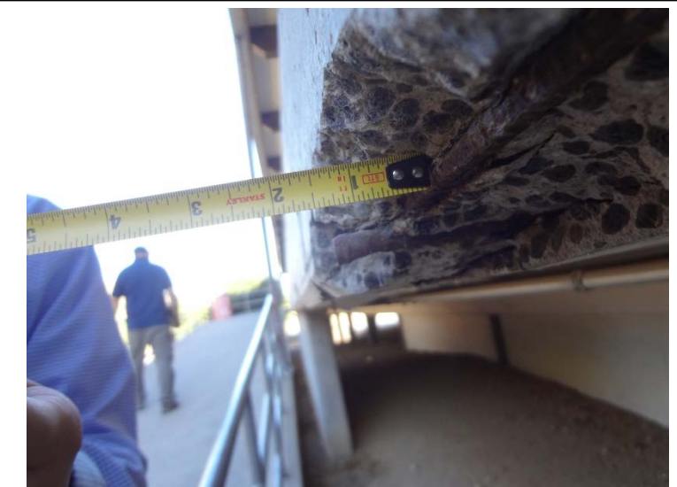
Photo -8 Elevated Classroom Walkway Spalling Concrete spalling occurs throughout the perimeter of balconies.
